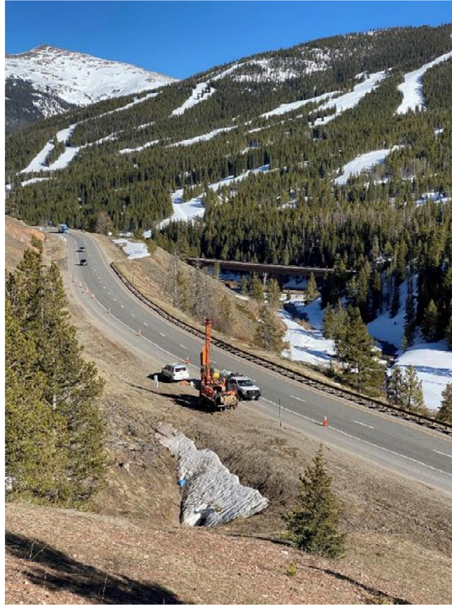
Figure 2. Area 1, Boring B-1 location near existing drainage. Eastbound I-70 bridge near Copper Mountain Ski Area shown in the background, looking southeast.
